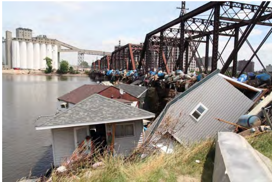
Union Pacific Railroad Bridge in Cedar Rapids during June 2008 flooding. Photo by Federal Emergency Management Agency
