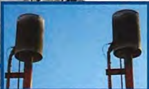
Building 99 Waste Gas Burners. Will be used as backup.
