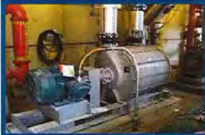
Building 75 Blower Room. Connection points for gas piping to/from biomethane system & various gas usage equipment
